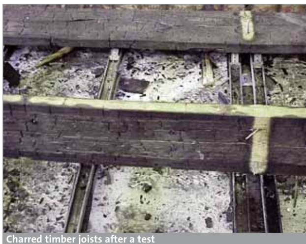
Charred timber joists after a test
